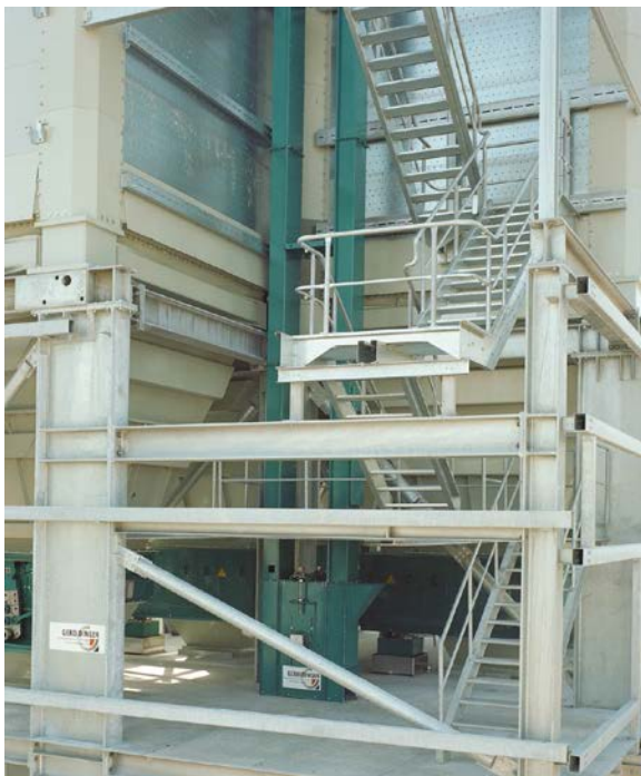
elevator buckets hardly show any wear
