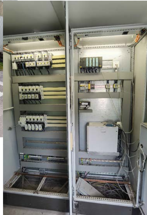
main control system of the silo plant
